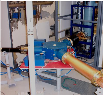
Klystron and Circulator
