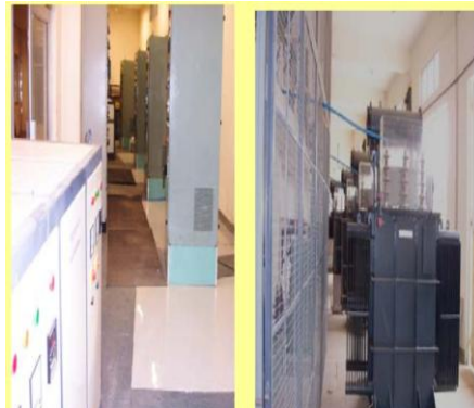
High voltage DC power supply
