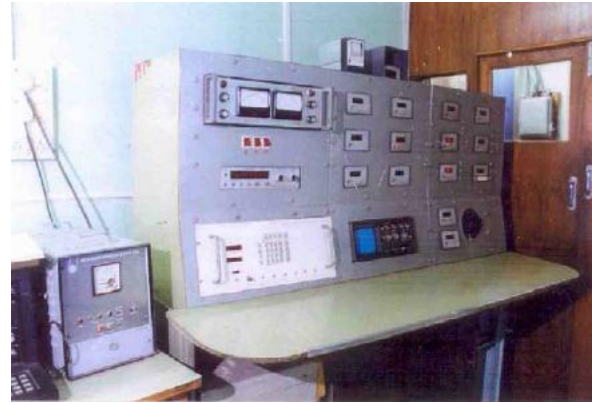
Figure 2: Control panel of the ion accelerator/14 MeV neutron Generator.
