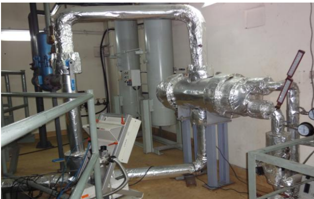
Fig.3. New SF 6 Chiller.
