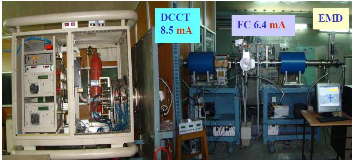
Figure 3: Ion source on high voltage deck and LEPT. Added to the system is fluorescence beam profile measurement device, diagnostic box two CCD cameras and associated software. At the end of beam line we see locally made water-cooled beam dump cum faraday cup.
