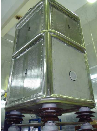
Figure 1: High voltage deck.
