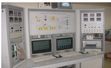
Figure1: Cryogenic control room at IUAC.
