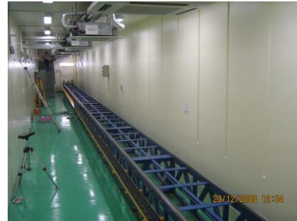
Figure 5: Calibration Lab with Ceiling Supply Air Units
