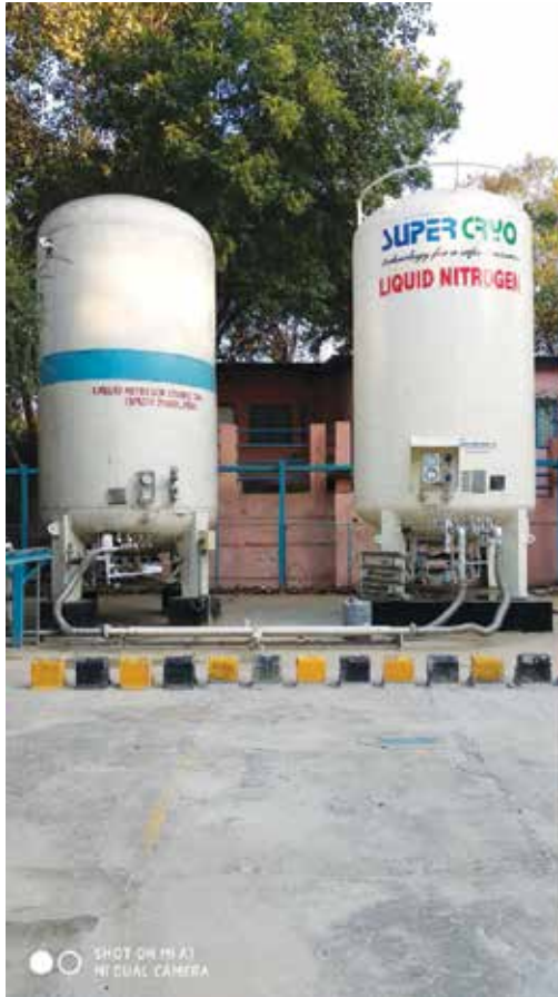
Fig. 3.1.7: 20000 lts LN 2 tank Total ext. capacity = 40000 lts
